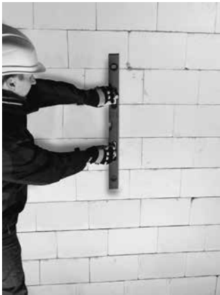
Image 18 Use a level to set out the path of the AMAXPRO soil and waste stack.
