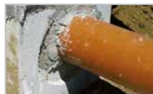
Leakage (in the long term)
